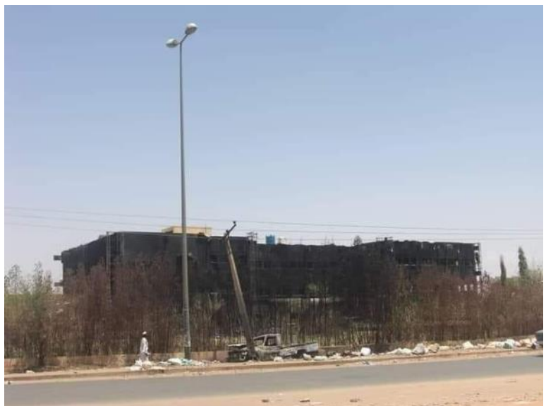
Image: IRCC (Industrial Research and Consultation Centre) building after it has been burned.
